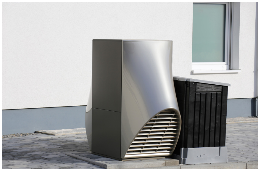
Example of a design that prevents optical noise and makes the heat pump almost invisible.
